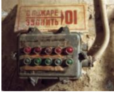
Bunker 42 Control Panel
